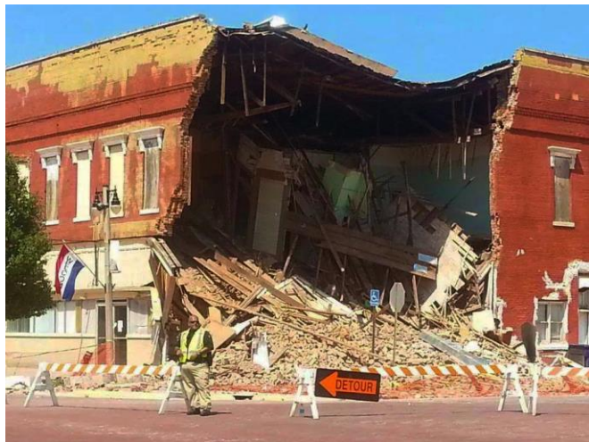
Picture 1: Building collapse, City of Kingman
