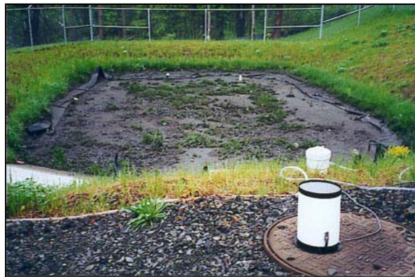
Figure 3-28 Sand Filter Example
