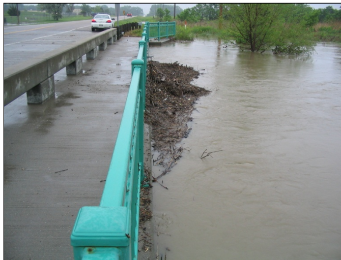
Figure 1-10 Trash and Debris at a Bridge Harry Street Bridge
