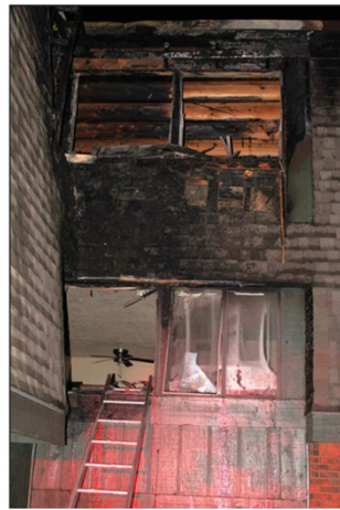
Figure 10: Post-fire damage to the exterior of Building 300. Living room windows seen for Units 306 (top) 304 (bottom). (Credit: WFD FIU)
